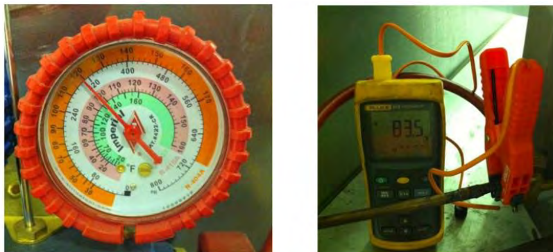
Figure 8 – Gauge Connection/Readings Liquid Line
