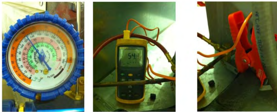
Figure 9 - Gauge Connection/Readings Suction Line
